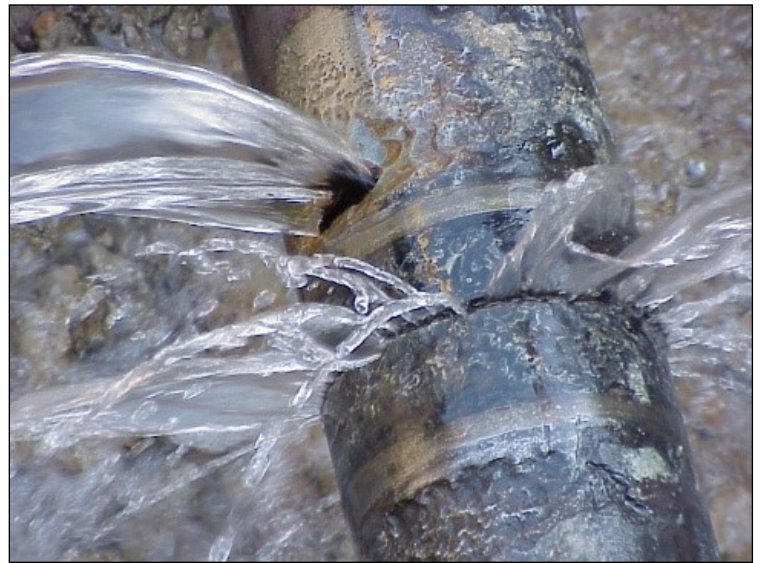
Water leaking from a supply line
