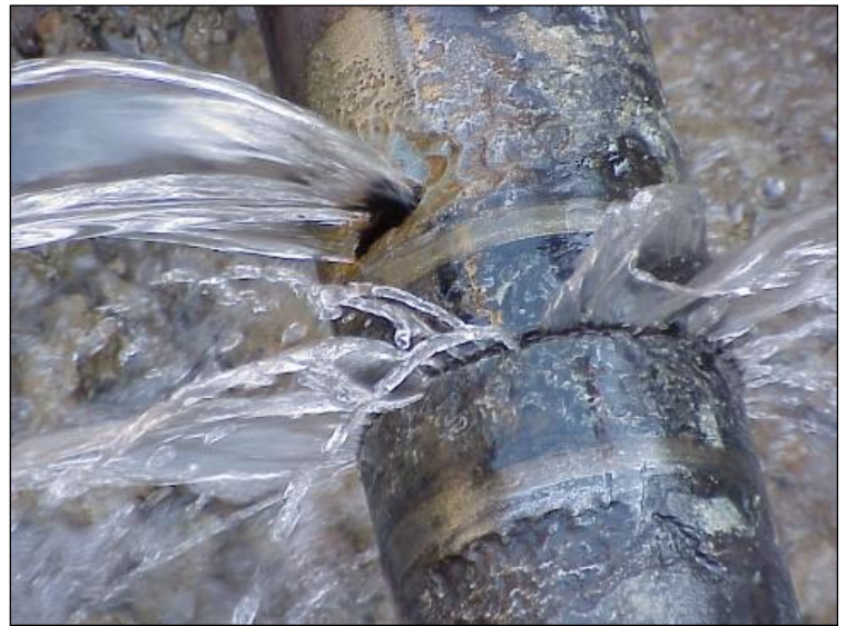
Water leaking from a supply line
