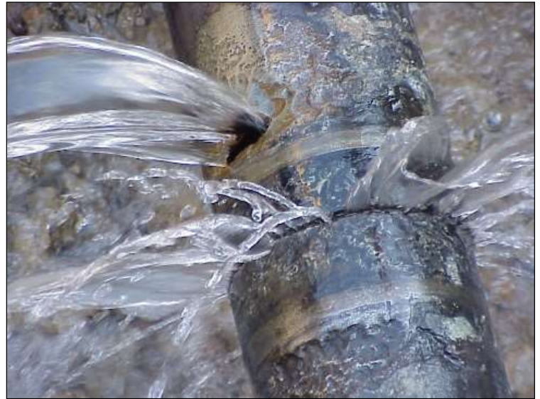
Water leaking from a supply line
